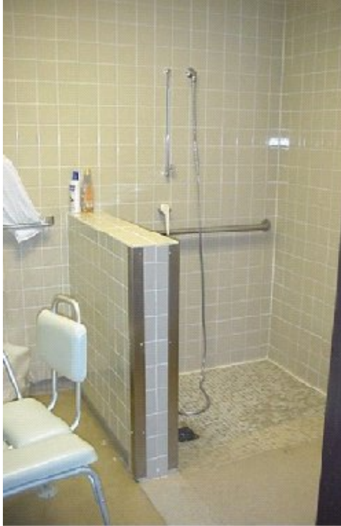
A half-wall on one side of the roll in shower can provide a shield from the water for someone who is helping bathe.
